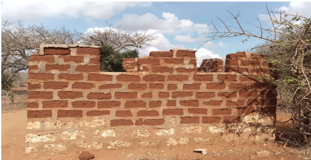
The unroofed toilet facility.
